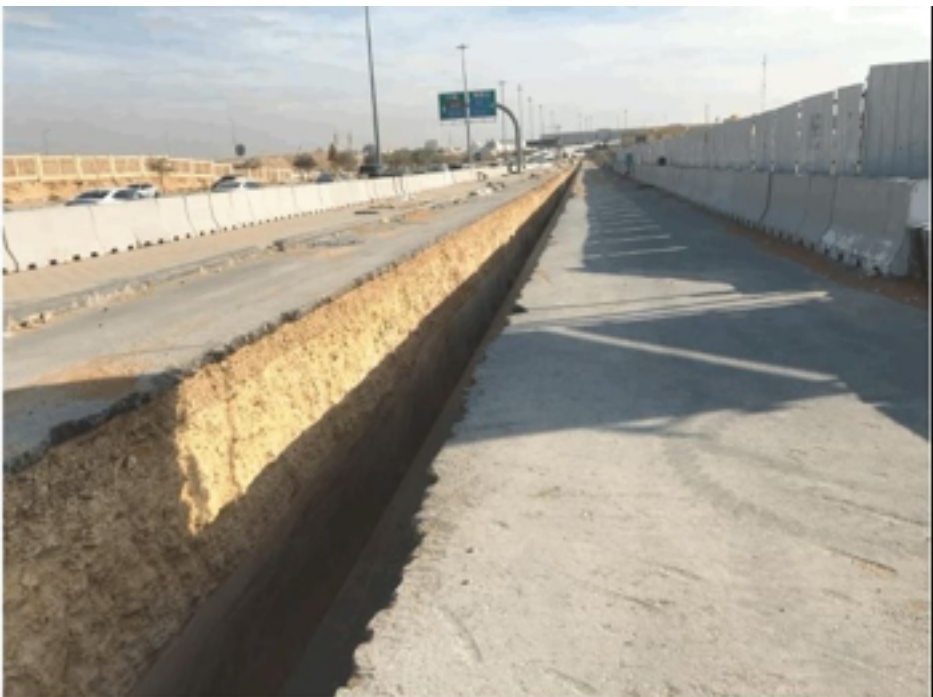
Unstable pipe and utility routes
